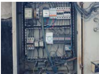
Electrical switchboard panels
