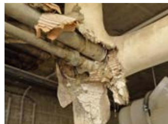
Pipe and duct coverings
